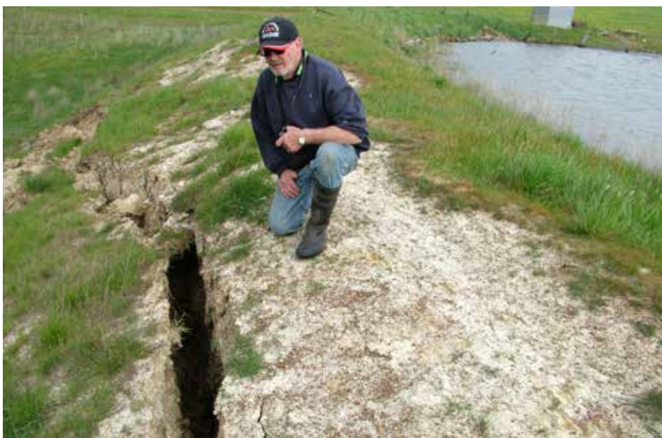
Peter Oddie inspects a crack in the back of a large dam on the family property at Ballyrogan
